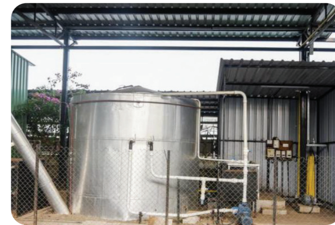
Biogas plant at Restaurant
